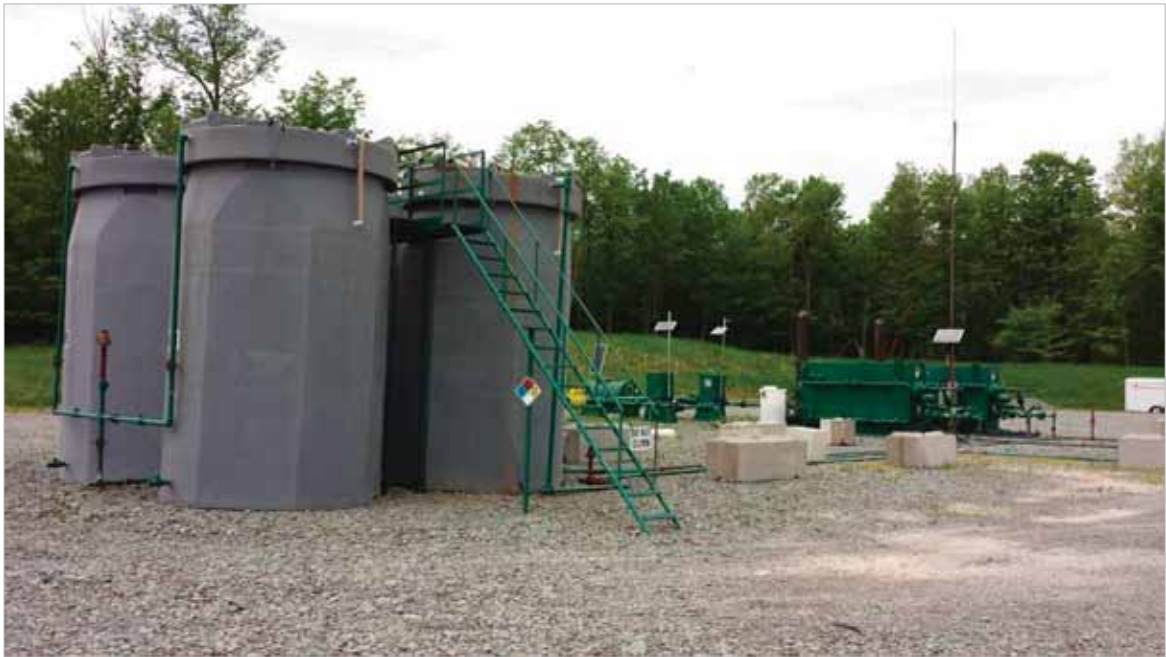
Figure 16. Remediated onshore shale gas well on private land in Dimock, Pennsylvania (from different angles) [Source: Committee site visit, 27 May 2014]
