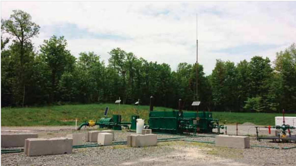
Figure 15. Remediated onshore shale gas well on private land in Dimock, Pennsylvania (from different angles)
