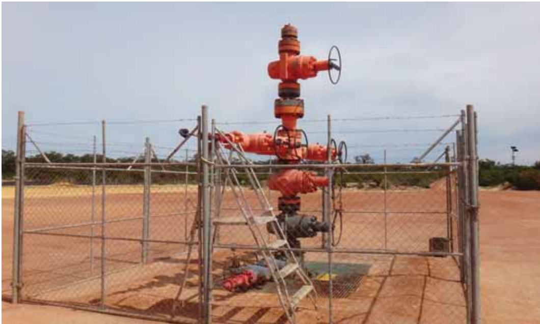
Figure 28. Christmas tree at decommissioned Arrowsmith-02 well [Source: Committee site visit, 28 October 2014]
