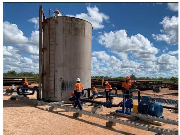
Produced water injection facility
