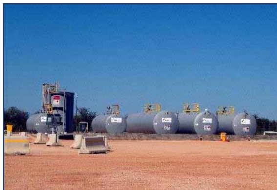
Ungani Field Facilities
