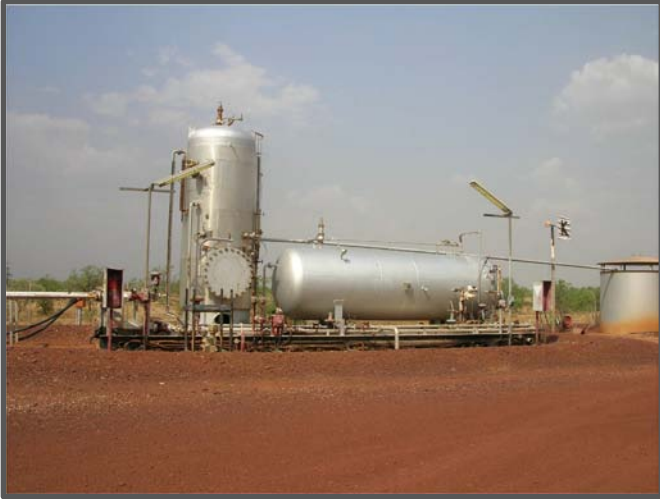
Blina oilfield facility
